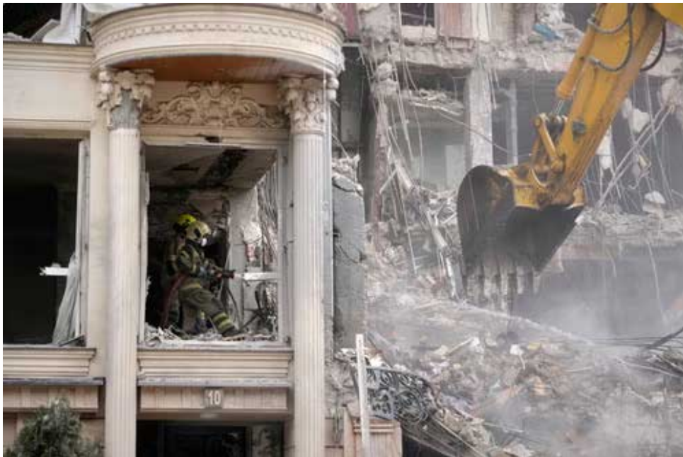
Rescue workers and first responders work at a residential building hit in an earlier US-Israeli strike in Tehran (AP)
